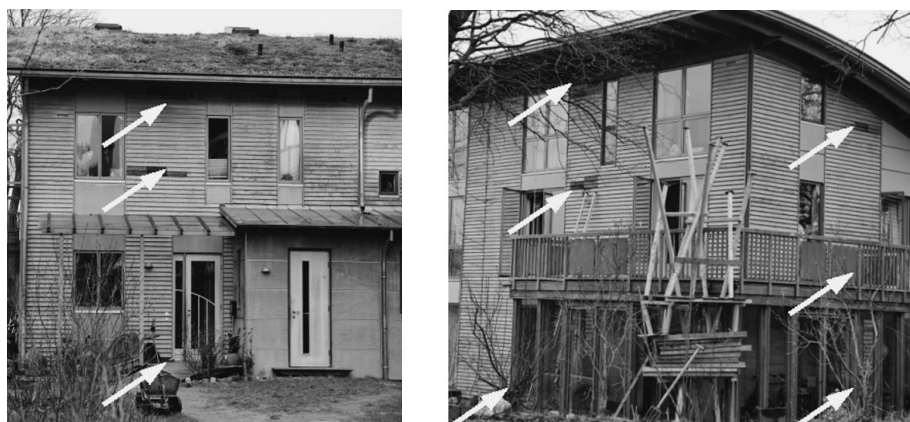
Figure 1 East and South-West orientation of the house facade in Kiel; Arrows point to the location of TMT boards with glued-in electrodes for long-term moisture recording
